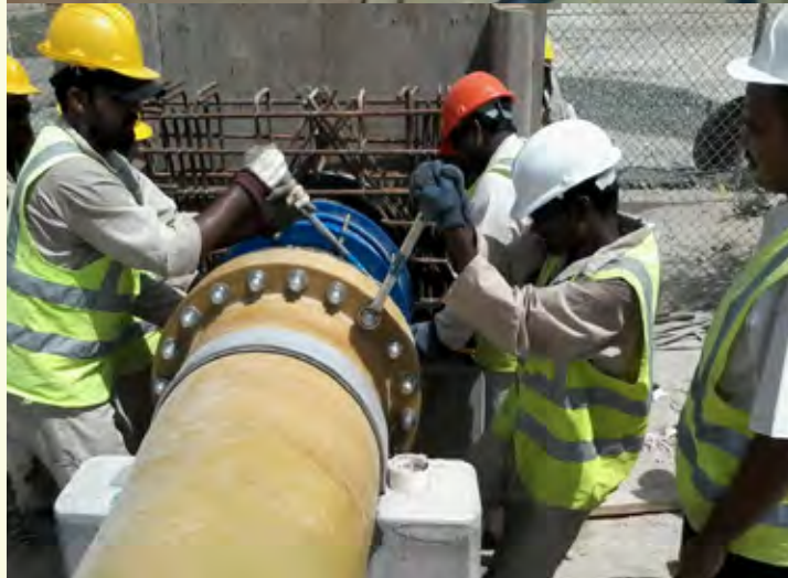
▲ AT WORK Skilled workers tighten the bolts on a flanged adapter under the specialist's supervision.
