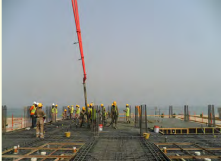
▲ ROOF SLAB Casting of roof slab is underway. Concrete pump is ready to start mix delivery.
