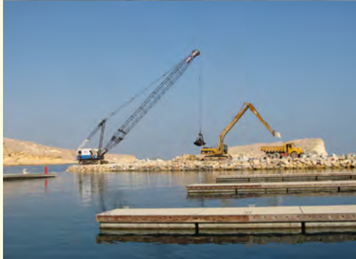
▲ MAIN MARINA BREAKWATER The team are seen working on the main marina breakwater. Special silt curtain was installed to protect the corals during the works.
