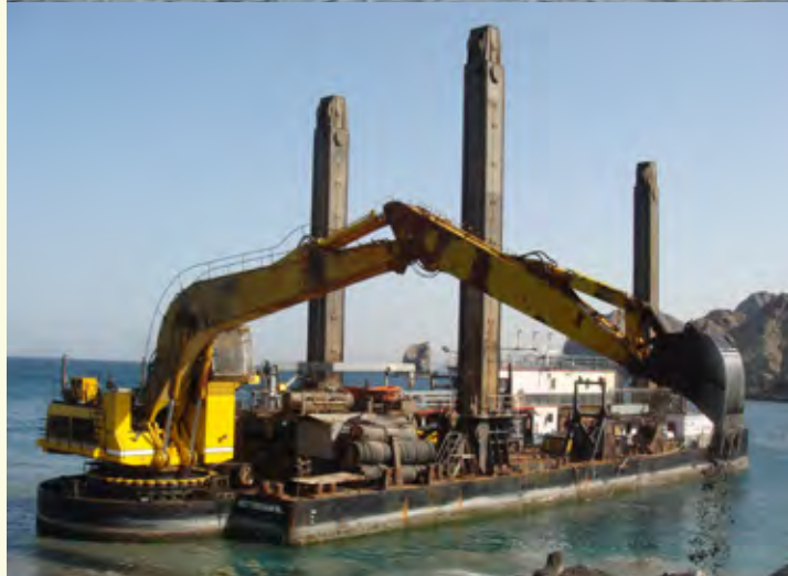
▲ DREDGER AT WORK Dredger "Ave Cesar" was mobilized to carry out the excavation works under water. It is seen here removing debris of previous revetment damaged by Cyclone Gonu
